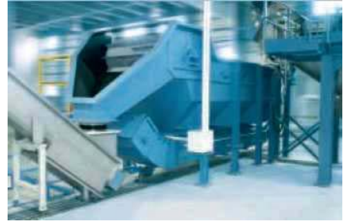
Flotation tank with scrape conveyor
