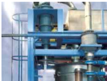
Part of a hydrocyclone plant
